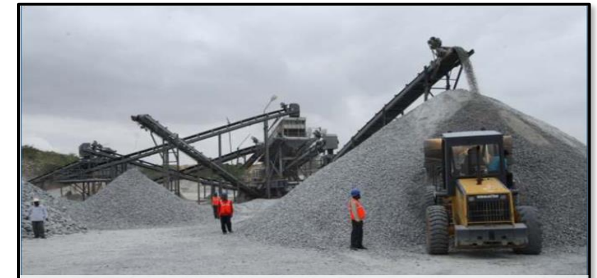
250 TPH Nawa Crushing Plant
