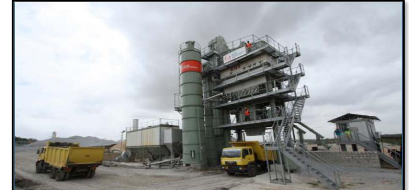
240 TPH D & G Hot Mix Plant
